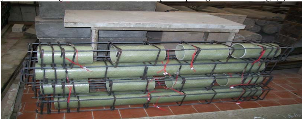
Fig. (1): GFRP Tubes and Rings Placed Inside the Reinforcement Cages. (Four Columns Stacked Horizontally on Top of Each Other Are Shown)
